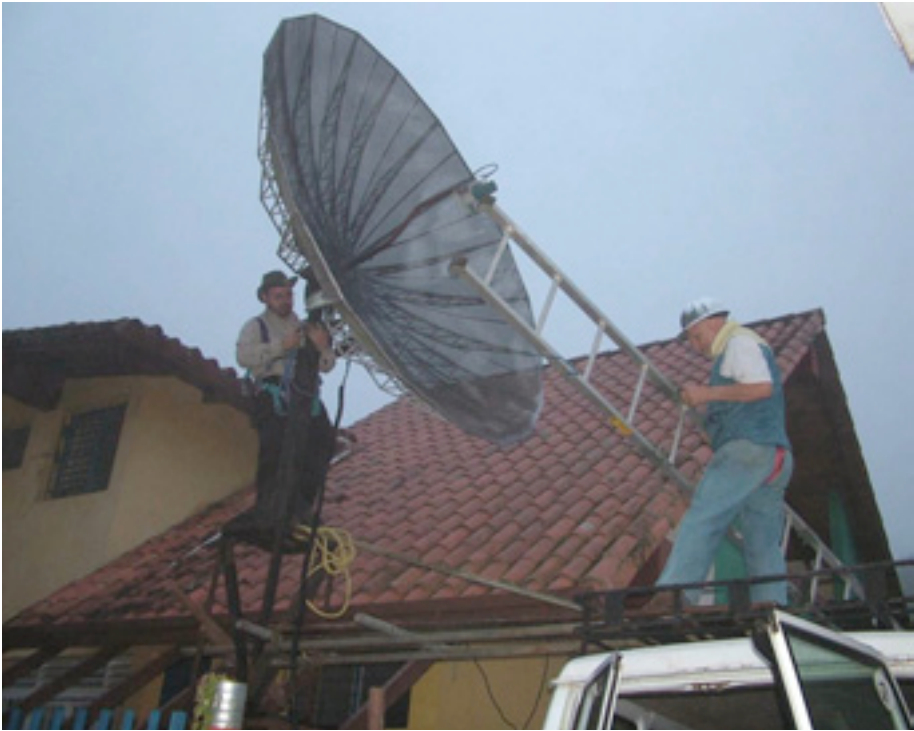
Figure 11.30: Carlo and Ermanno disassembling the satellite dish supplied by Mr. Ismael Santos.
