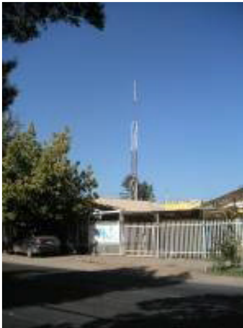
Figure 11.21: Node in southern Santiago, consisting of a 15 m tower, a Trevor Marshall 16+16 antenna, and 30 clients. The node is connected to a downtown node more than 12 km away.
